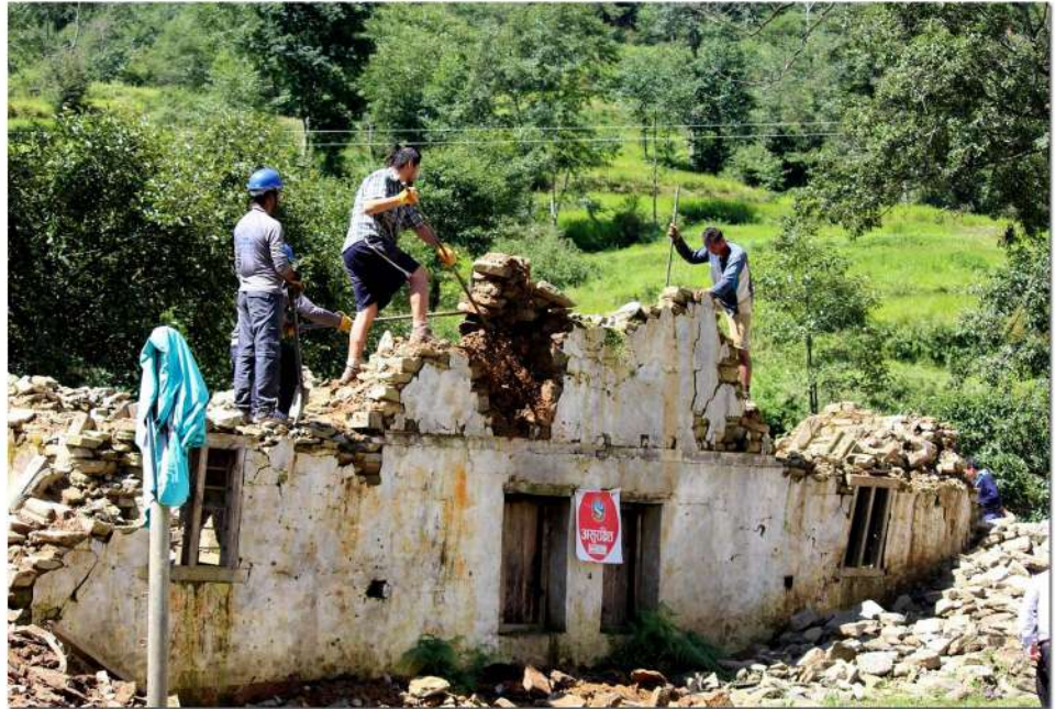
Photo 8: Work Camp Volunteers breaking down a dangerous section of a Buddhabhimeshwori Secondary school, Mali destroyed by the earthquake in Dolakha
